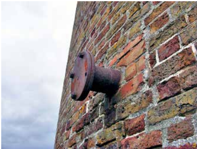
One of the two FSM pipes protruding from the tower wall. Photo Mark Russell
